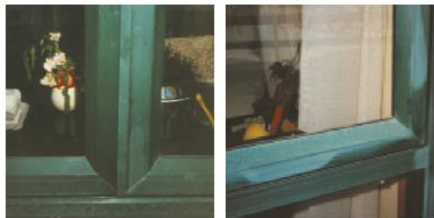
Examples of solvent misuse on aluminium joinery, showing deterioration of powder coating after 3 years.
