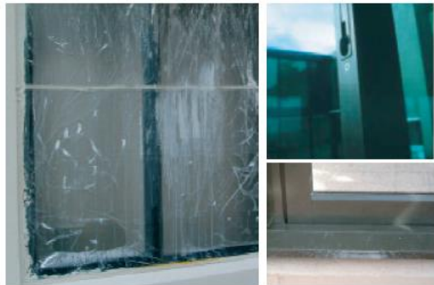
Three of these photographs display damage that has occurred on site, post installation. The photo of the masked joinery on the left displays clear signs of damage that could have occurred were it not masked. Please ensure that your joinery is protected right through the entire construction process.
